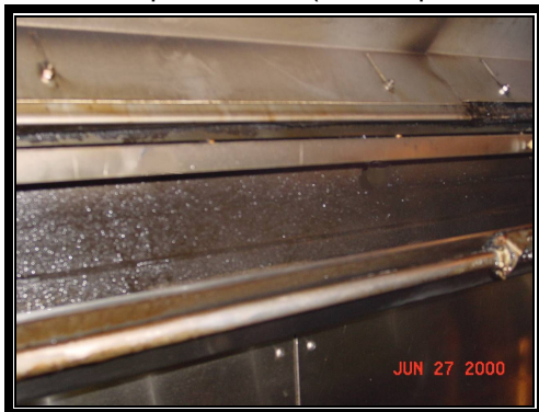
Inspect Baffle Positions
