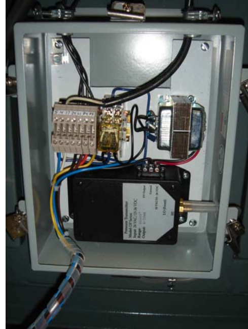
Inside the MXFLOW L20 panel Figure 28
