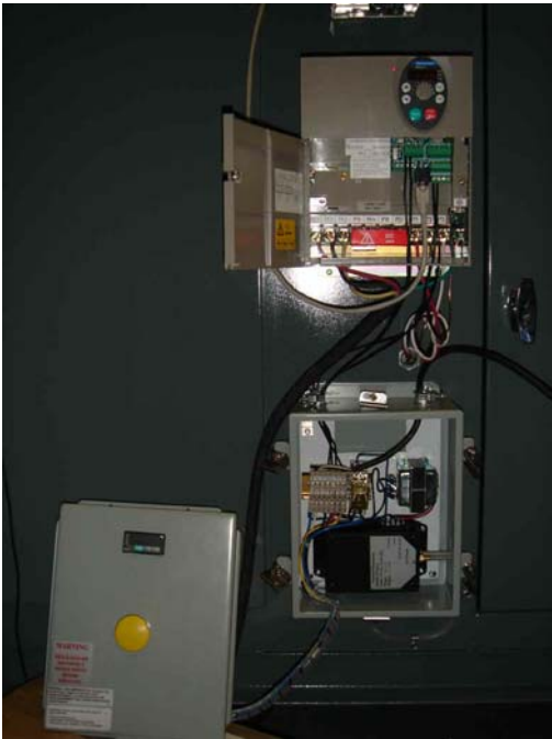
Variable Speed drive and LV20 panel mounted on side of the KESF unit.
