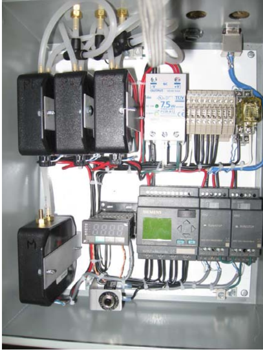
Inside the LV10 panel with MXFLOW Figure 28
